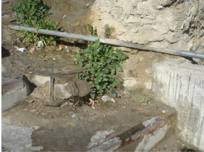
Figure 17: Sewage issues in al-Moghrabi site
